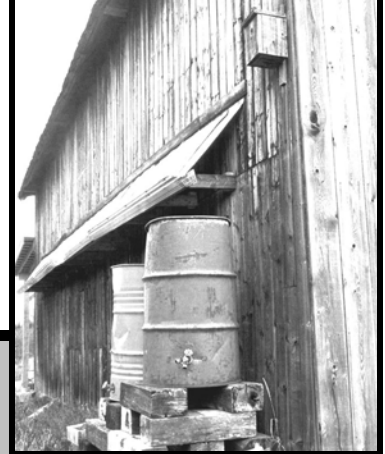
Rain barrels at work at Falls Brook Centre, NB
